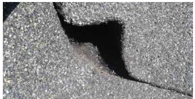
Leakage in an overlap
