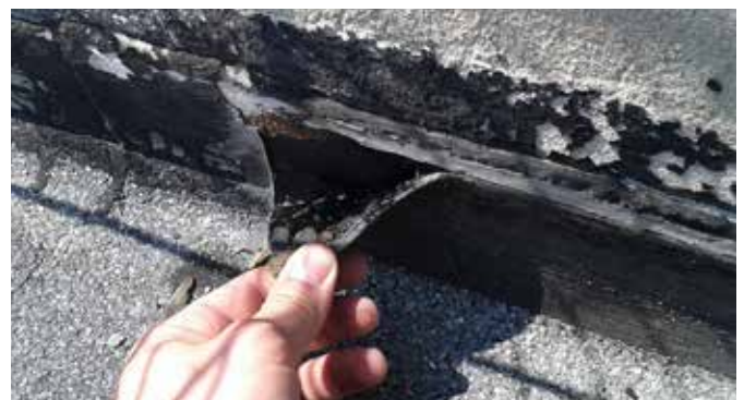
Damaged chimney flashing
